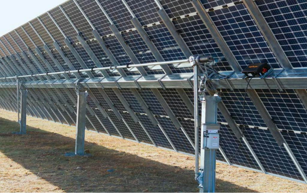
STABLE AT FLAT STOW Nextracker’s 2P NX Gemini tracker—shown here at the National Renewable Energy Laboratory’s (NREL) Flat Irons Campus for wind testing in Boulder, Colorado, U.S.A.—incorporates self-locking linear actuators at each foundation to ensure stability against dynamic wind effects.
